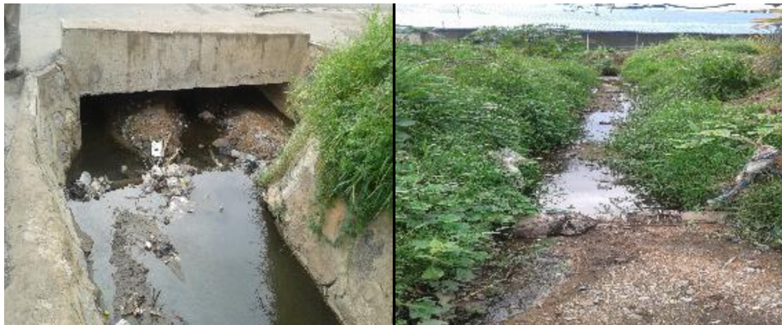
Figure 4.4: R: Silt accumulation under the Igogo VTC culvert. L: Downstream side of the Igogo VTC drain
