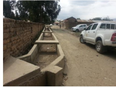
Figure 5 Inadequate drainage structures for storm water outside the fence of TECU in Mwakibete area
