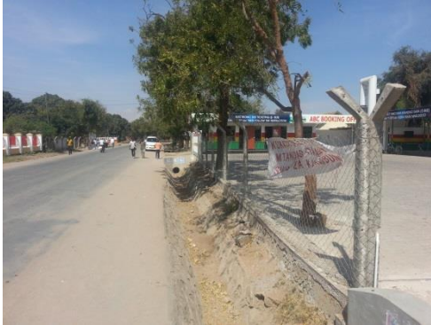
Figure 3: Drain for improvement outside Main Bus Stand
