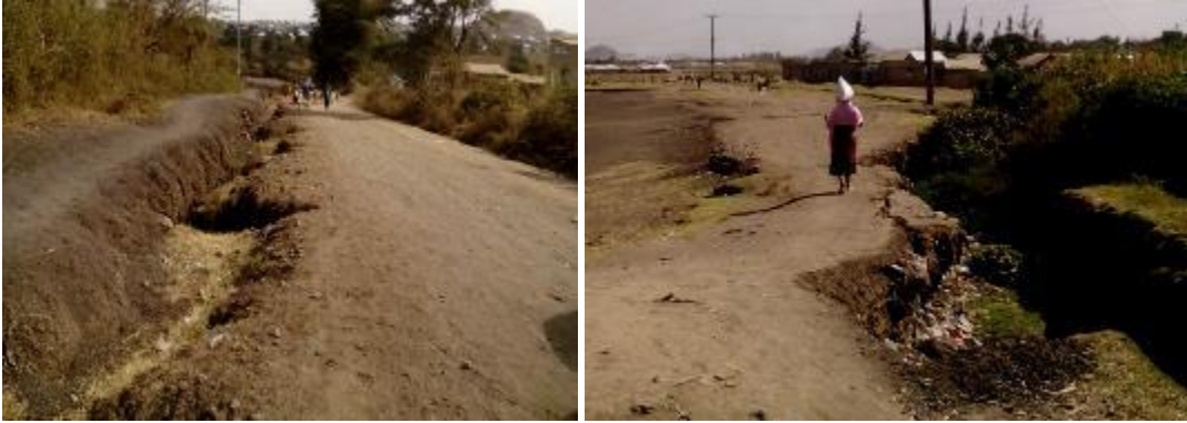
Figure 4.3: Areas along the road affected by floods and erosion
